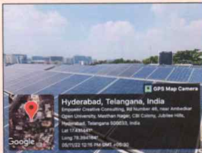
Photograph of Solar Thermal Water Heating System: at Yash Inn Facility
